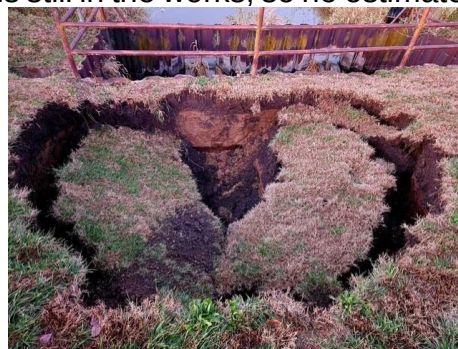
Collapsed culvert on Beaver Lake Blvd
